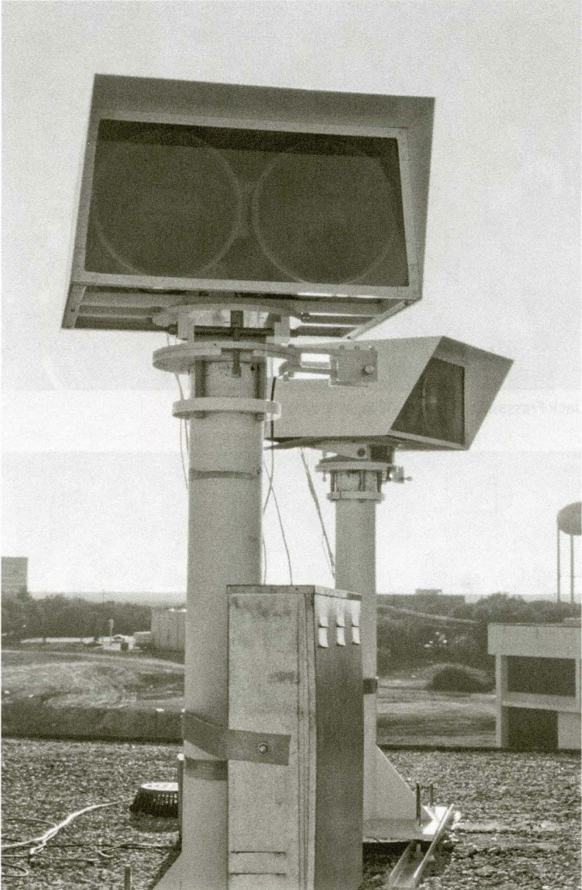
Production Datapoint LightLink Infrared data transmission system installation
